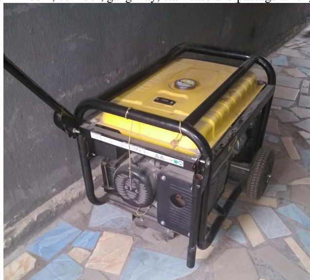
Figure 2: Generator in a corridor
