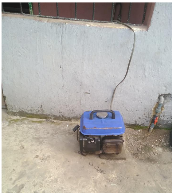
Figure 3: Generator in close proximity to house
