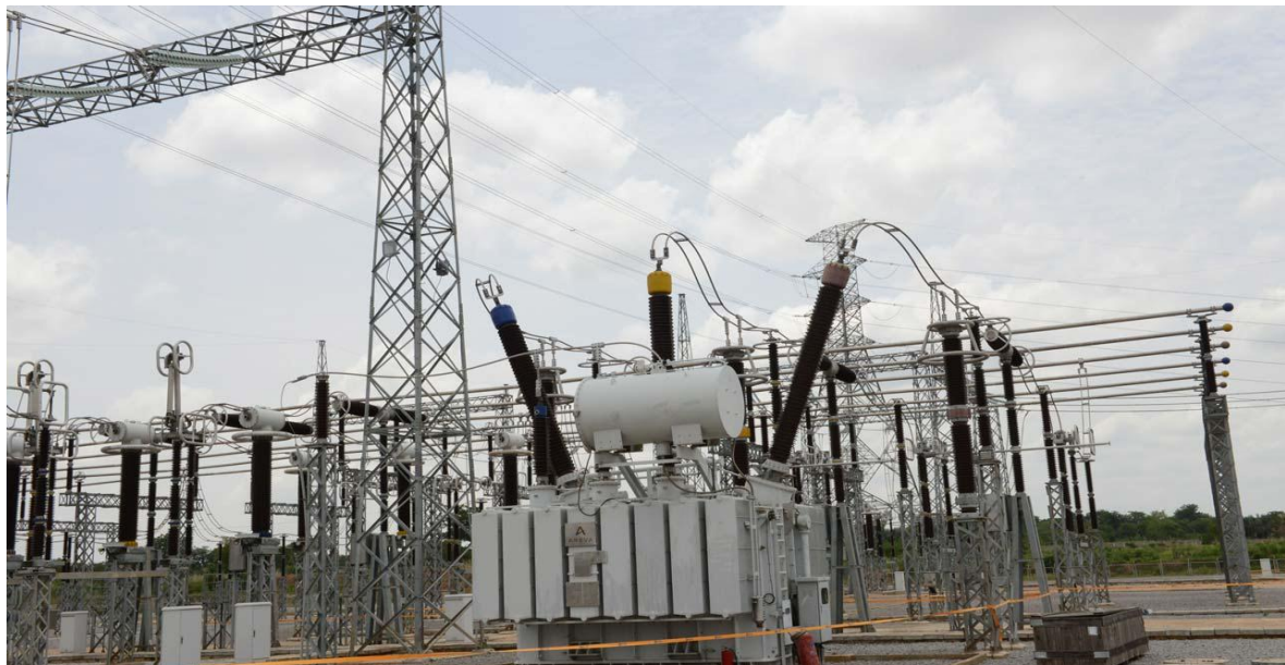
Fig. 2: Pictorial view of Nibo substation, Awka South L.G.A, Anambra State
