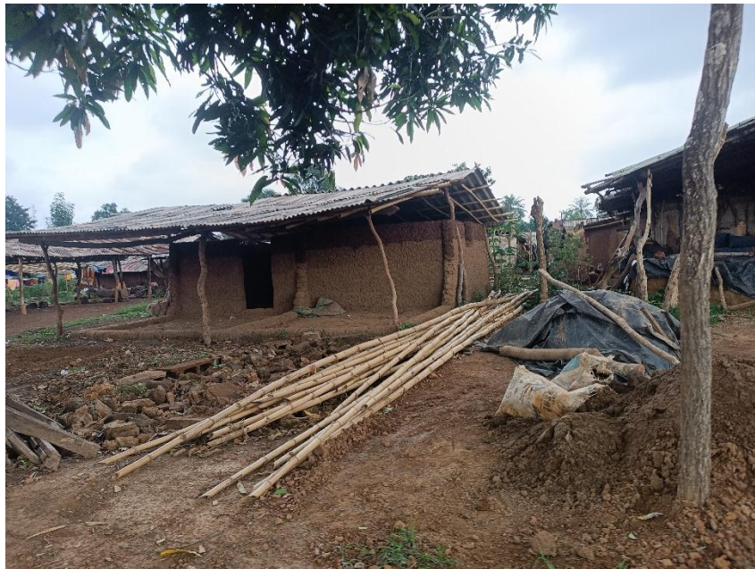
Plate 2: Pictorial View of bamboo used as roof members. Source: Author's fieldwork; May 2024.
