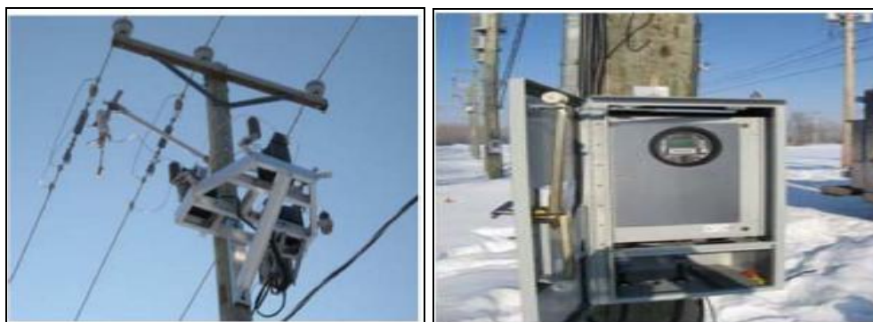
Fig 3: (a) Capacitor bank
