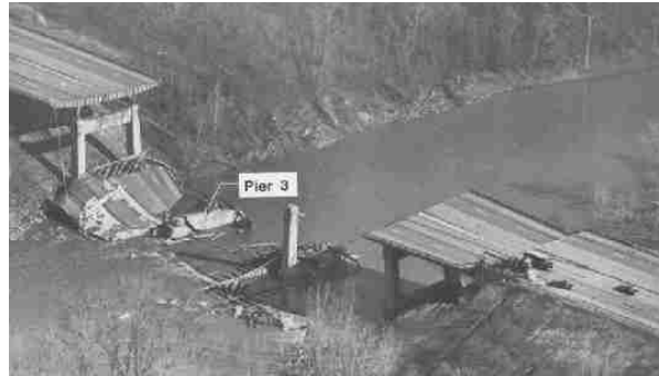
Fig. 1. Photo of schohaire Creek Bridge April 5, 1987 (Courtesy of the National Bridge Inventory Web Page)
